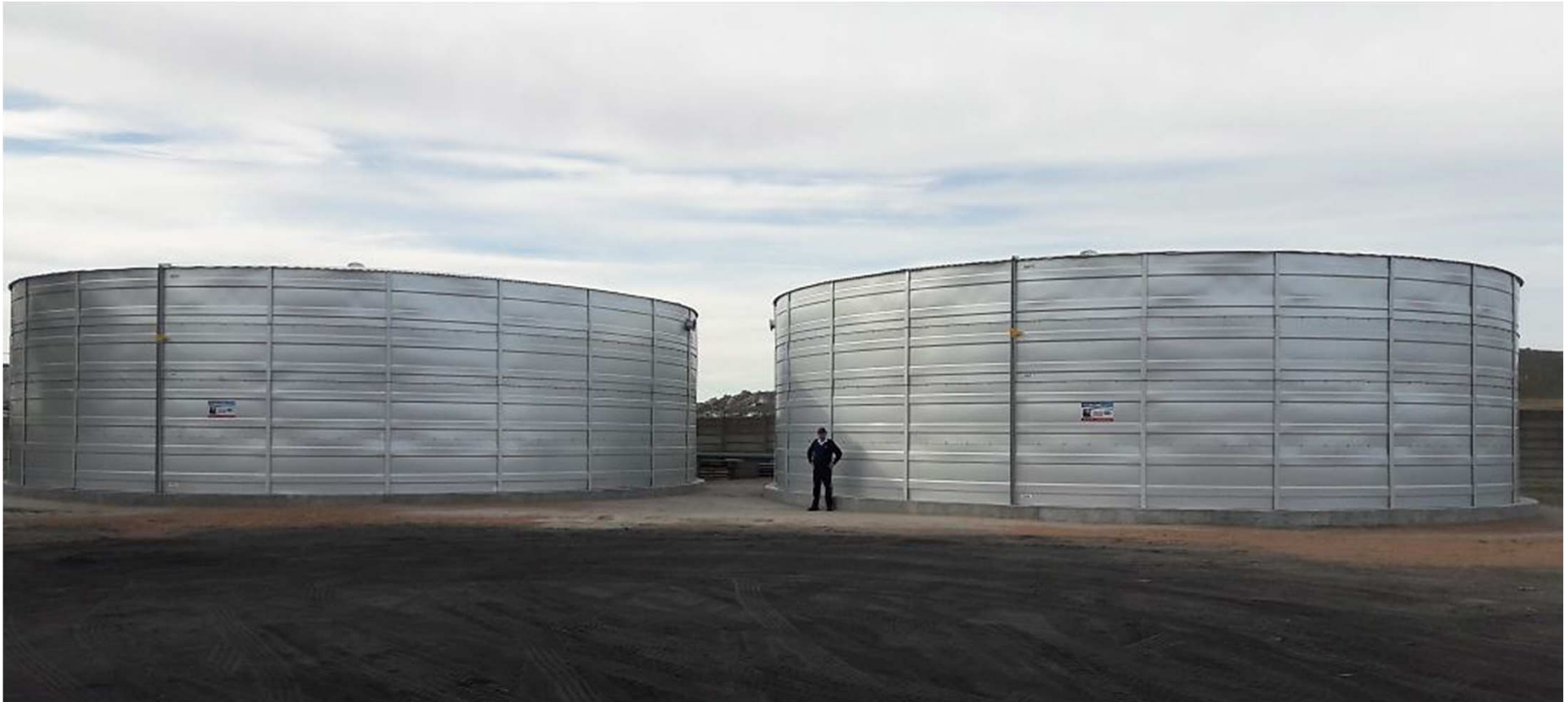
2 X 1 MILLION LITRE TANKS AT ST HELENA BAY
